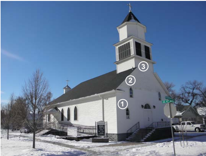
Gothic Revival Church - 404 11th St., ca. 1918 - Greeley Historic Preservation Office, Colorado State University interns, 1/13/2011 (non-historic siding)
