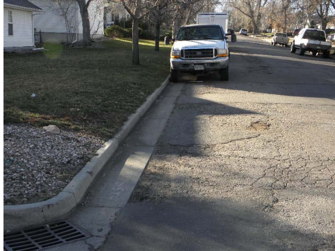
12 St. & 16 th Ave.- Missing sidewalk and access ramp
