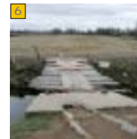
Existing crossing over Greeley no. 3 ditch. Would need to be upgraded to accommodate trail.
