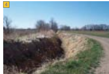
4 West ditch rider road along Boomerang Canal near US 34 looking southeast. Trail will be along east ditch rider road.
