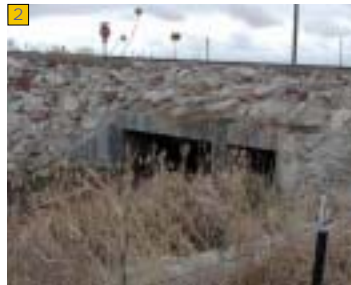
2 Sheep Draw crossing under 95th Ave. Significant improvements required to accommodate trail underpass.
