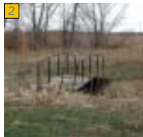
Existing private bridge crossing. If alternate alignment is selected to pass through this area, this point provides the easiest crossing.
