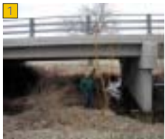
Existing 4th St bridge does not seem to accommodate a trail bench without re-grading, creating a trail bench and crossing the drainage. The channel has no definite path under the bridge.
