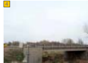
Existing bridge at 37th St. should be able to accommodate a trail underpass with minimal improvements.
