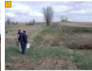
5 Trail crosses side channel along fence line. A culvert and upgraded pedestrian crossing will be needed.
