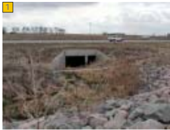
1 Sheep Draw crossing under US 34. Significant improvements, ie. new taller box culvert, slope and grading required to accommodate trail underpass.
